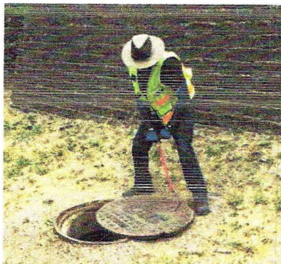
Carefully open the facility lid using a manhole puller. Look inside the structure from above. Look for cracks, sediment, trash, and dirty water. Do not enter.
